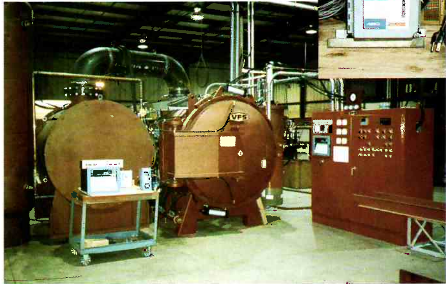
Fig. 1 Electrolytic hygrometer is utilized for measurement of moisture in operation of a vacuum heat treating facility. Inset shows closer view of the hygrometer.
