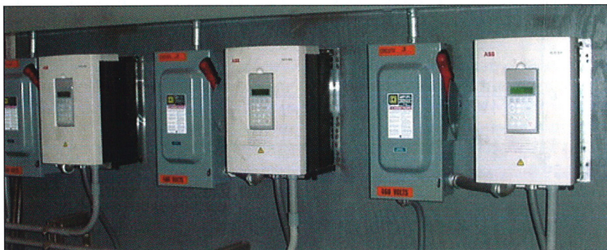
Fig. 2 — Variable speed drives automatically control motors of water pumps to deliver lowest possible electric cost.
