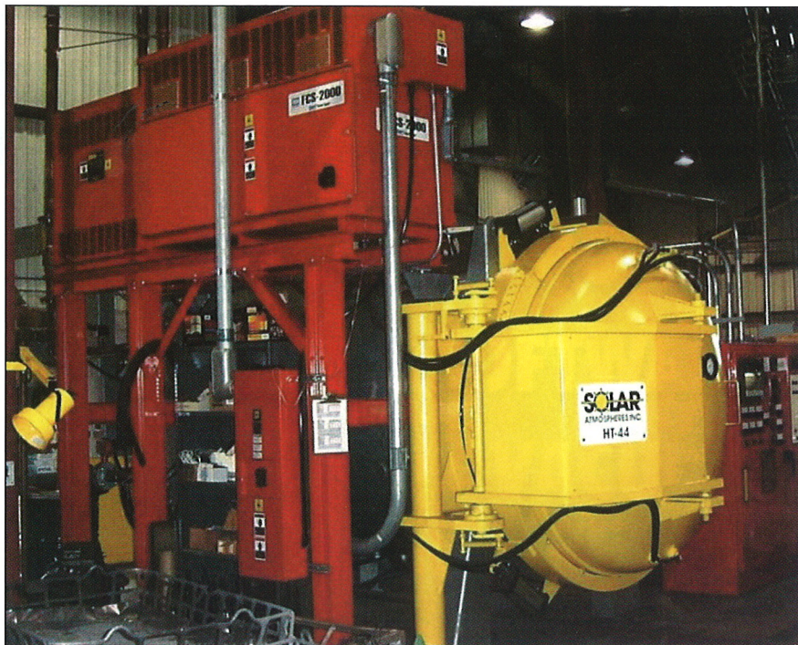
Fig. 9 — Installed on a vacuum furnace with graphite heating elements, a 255 kW smart power supply (FCS-2000) combined with a tapped power transformer has operated for more than 10,000 hours.
